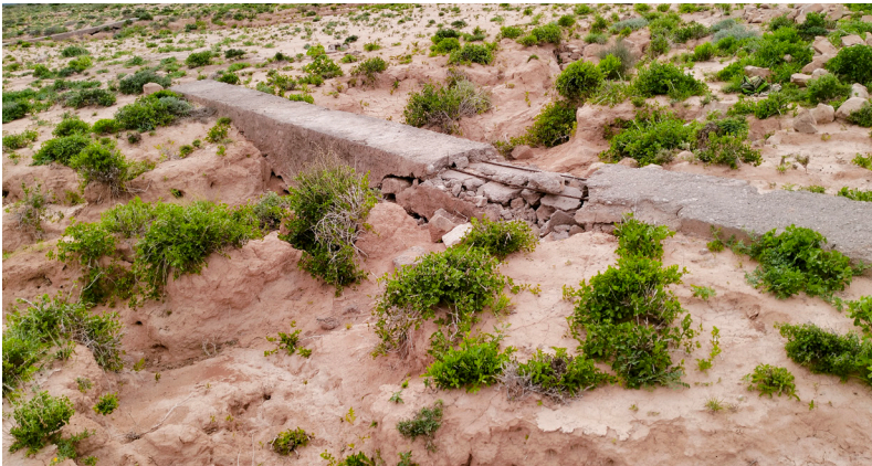
Figure 8: Damaged check dam.
