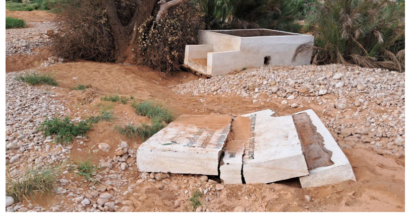
Figure 3: Damaged Shallow well.
