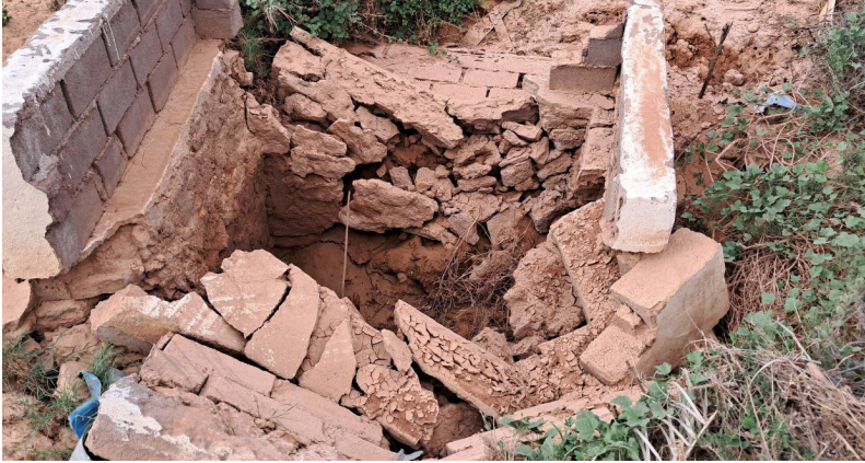
Figure 2: Destroyed Shallow well.
