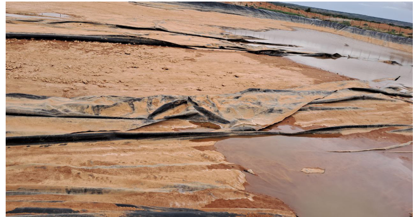
Figure 5: Damaged HDPE sheet for the earth Dam.
